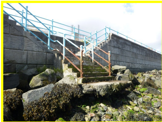
Undercutting of access steps (/C0401C27)
