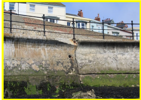
Damage to recurve concrete cope (/C0401C04)
