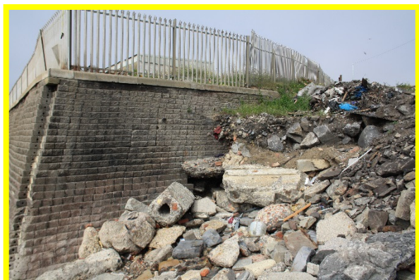
Scour hole and evidence of settlement visible at northern end of seawall (/C0401C19)
