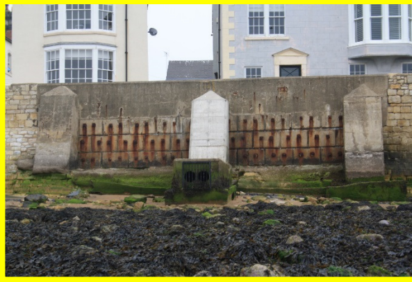
Recently constructed outfall and abutment. Significant corrosion/rust staining previously observed (/C0401C35)
