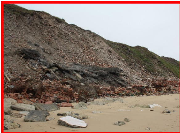
Collapsed former gabion structure (/C0302C02)
