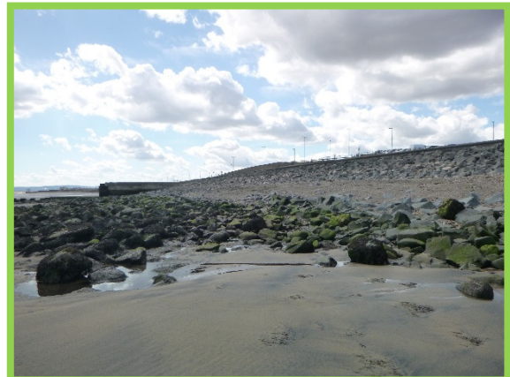
Possible displaced rock in foreground (/C0401C33)
