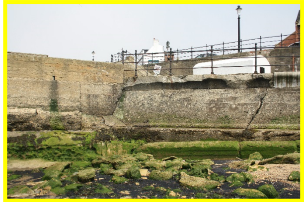
Spalling damage to recurve wall, significant crack suggesting settlement. Old Pier to left of image (/C0401C05)
