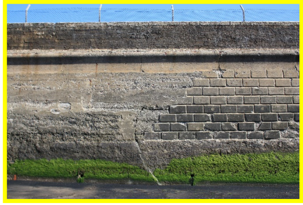
Vertical crack through parapet and seawall (/C0401C20)
