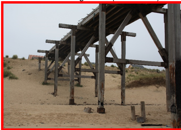
Loss of section to timber support columns of historic pier structure, likely due to fire damage (/C0302C01)
