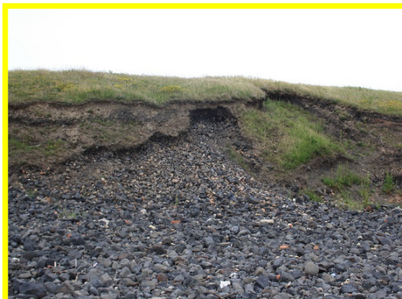
Local slope failure (/C0302C03)
