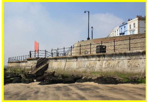
Low beach levels at access steps (/C0401C04)
