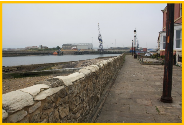
Heavily abraded masonry at crest of wall. In some areas mortar used in repointing appears to be stronger than masonry and stands proud of stone (/C0401C35)
