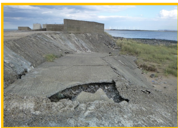
Voiding along south face of North Gare Breakwater (/C0503C01)
