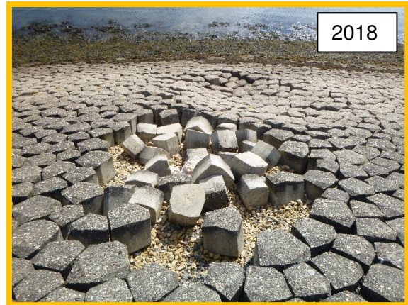
Local settlement of concrete blocks (/C0401C26)
