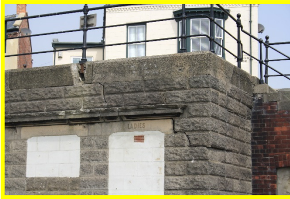
Cracking in former public convenience building (/C0401C05)
