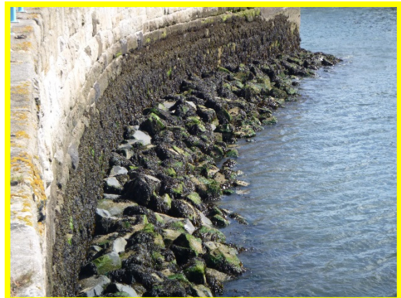
Outer face of Middle Pier – note profile of rock armour at seaward end (/C0401C28)
