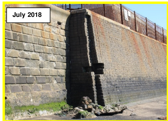
Progressive loss of blocks at interface between two walls. Local scour at toe (2018) (/C0401C19)
