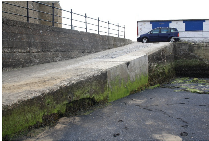
Recent concrete repair to slipway, voids/undercutting remains (/C0401C35)
