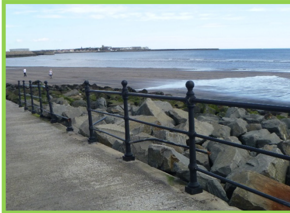
Displaced rock armour and damaged guardrail at northern access ramp (/C0401C33)
