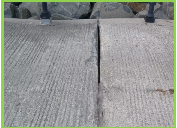
Loss of flexible joint sealant (/C0401C33)
