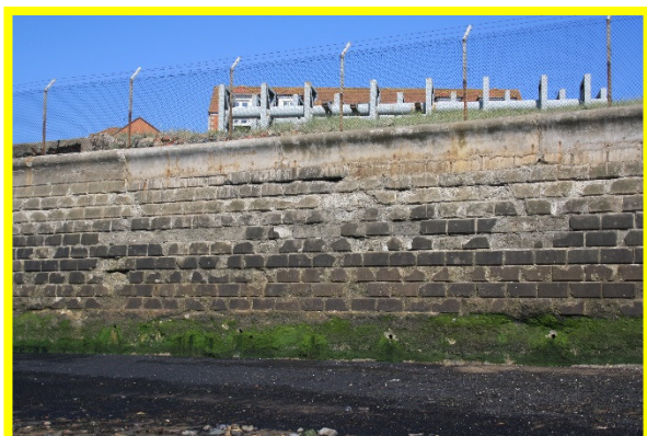
Spalling/abrasion of concrete blocks (/C0401C19)
