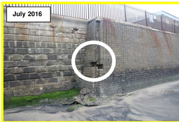
Missing blocks at interface between two walls. Local scour at toe (2016) (/C0401C19)
