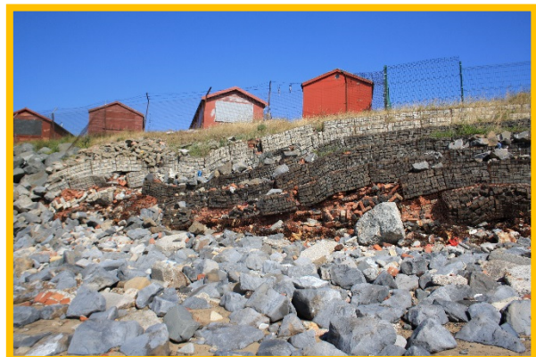
Settlement in stacked gabion wall (/C0401C17)
