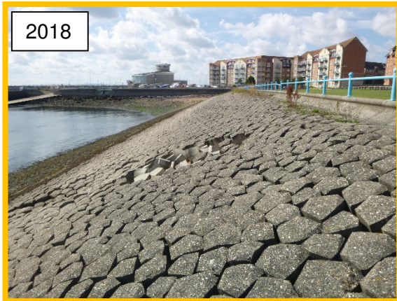
Local settlement of concrete blocks (/C0401C26)
