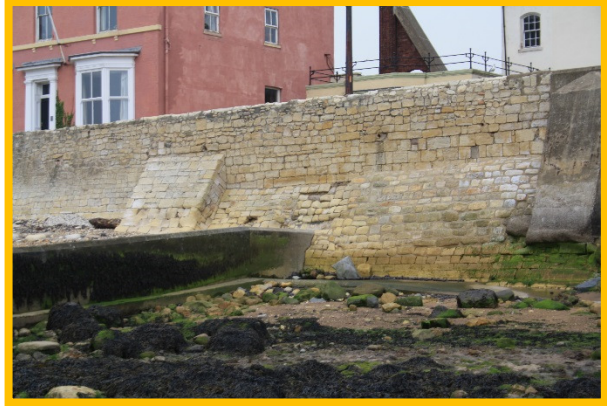
Open jointing in lower masonry courses. Local undermining of concrete buttress (/C0401C35)
