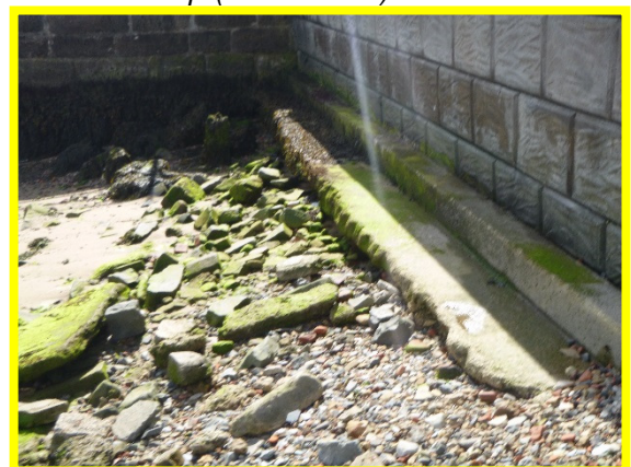
Low beach levels exposing undercutting of concrete toe (/C0401C27)
