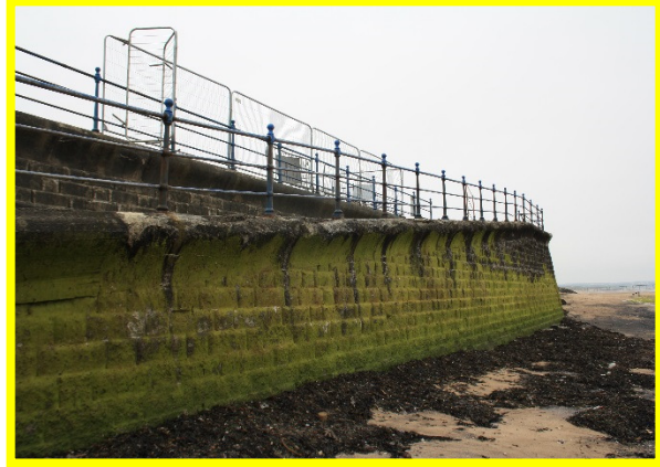
Local damage to coping/handrails at Arabella Street access ramp (/C0303C01)
