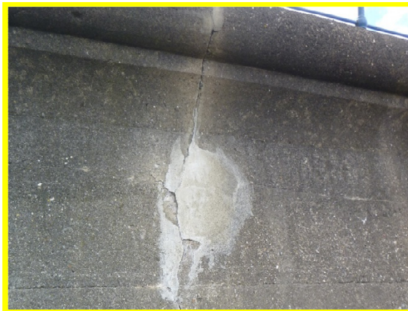
Local cracking and spalling of concrete (/C0501C05)
