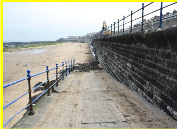
Access ramp at Arabella Street, previously undercut (/C0303C01)
