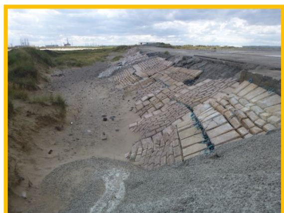
South face of North Gare Breakwater. Dune field in lee of structure (/C0503C01)
