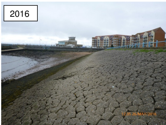
Local settlement of concrete blocks in 2016 (/C0401C26)
