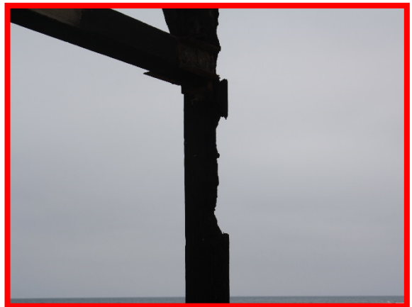
Loss of section to pier support columns, likely due to fire damage (/C0302C01)
