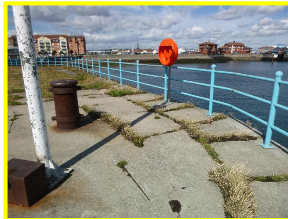
Extensive vegetation growth through joints in Middle Pier deck (/C0401C28)
