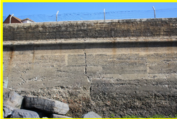
Vertical crack through parapet and seawall (/C0401C20)
