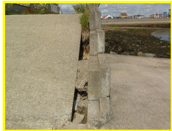
Void behind concrete wall units and beneath concrete ramp (/C0401C27)
