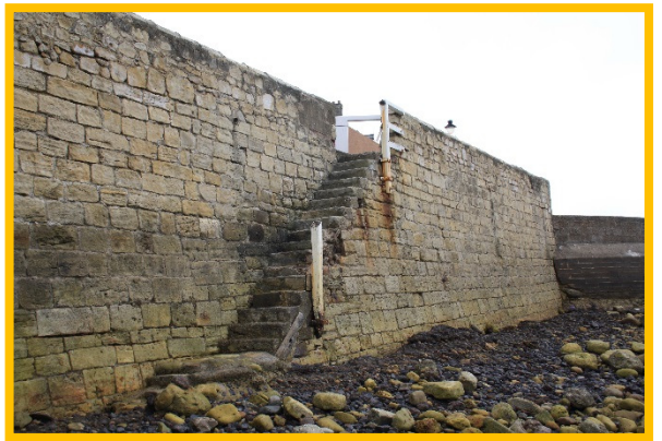
Several open joints in masonry (/C0401C35)
