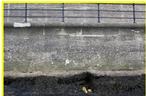
Void at toe of seawall obscured by marine growth (/C0401C05)
