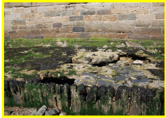
Voids in apron of North Pier, approx. 0.5m depth extending under concrete and through timber piles (/C0401C22)
