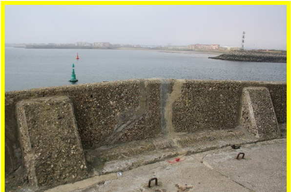
Cracks in concrete parapet wall and deck filled in with cement/grout (/C0401C34)
