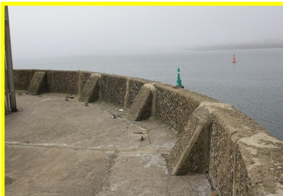
Cracking in parapet wall and deck, and gaps between 'buttresses' and wall filled in with cement/grout (/C0401C34)
