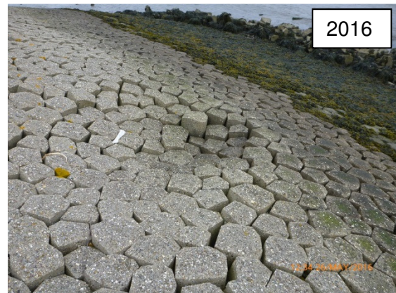
Local settlement of concrete blocks (/C0401C26)
